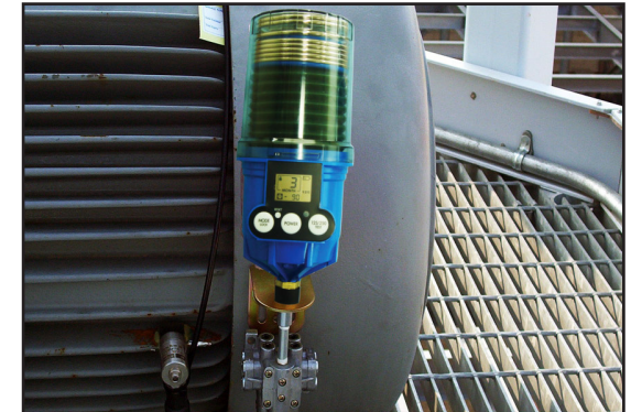
Safe, reliable, easy-to-maintain and service – helping to keep the university reliably cool.
