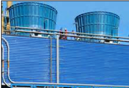
Forced downdraft cooling towers used by a major university for HVAC cooling water.
